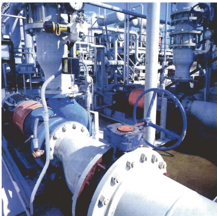
Fig. 1. Pumps that become a part of process control systems can improve plant operations.
